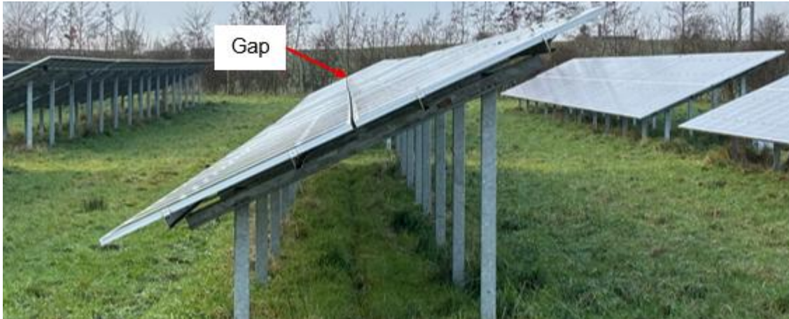
Plate 15.53: Solar PV Arrays Showing Gaps Between PV panels
