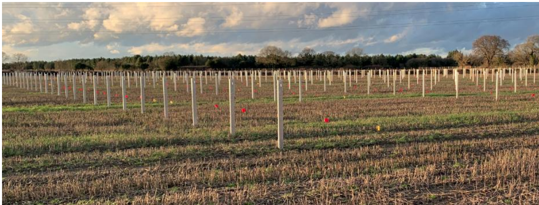
Plate 15.31: Mounting Structure Piles being Installed (taken at Tiln Farm, Retford, in January 2023)
